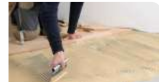
Cracking at corners & around cuts may be caused by improper conditioning, Improper bonding, poor planning.
